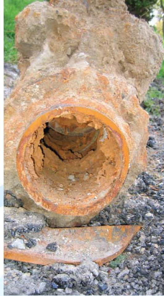
Aging municipal water distribution pipe.
